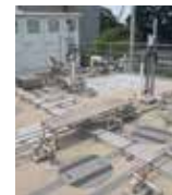
Wastewater treatment facilities
